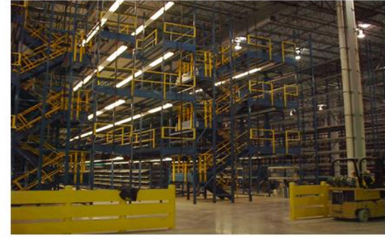
This four-level pick-module is the centerpiece for this #1 retail drug chain DC's recently completed in Texas, Ohio, and California .
